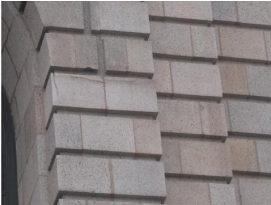
Figure 139: Detail view of terra cotta typical of the first floor level. Note the cracked units visible in the photo. Approximately 25% of the units on the building are cracked.
