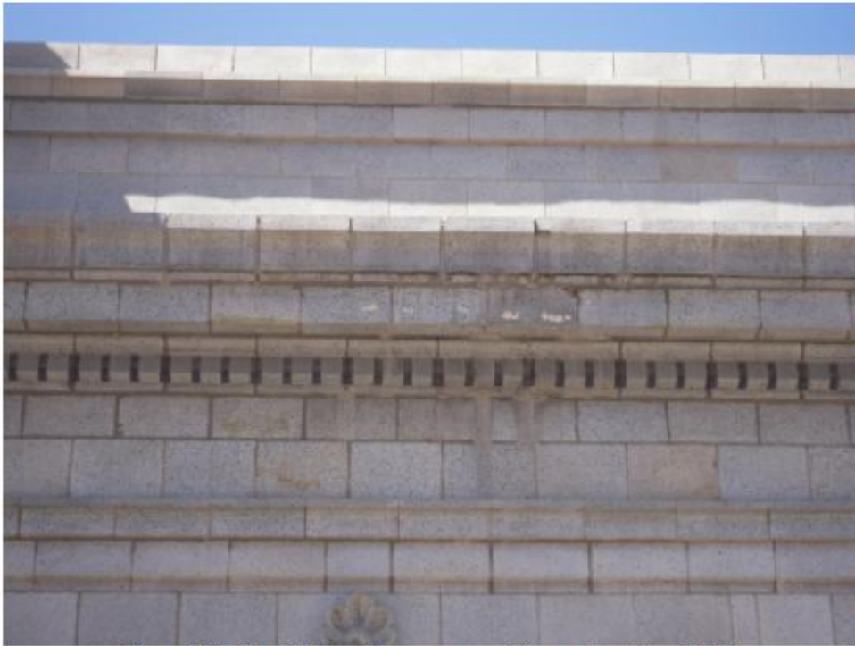
Figure 135: Detail view of terra cotta spalling at location of drain.
