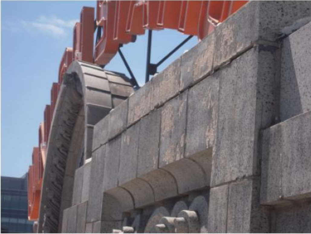
Figure 147: Detail view of terra cotta spalling visible below the sign.
