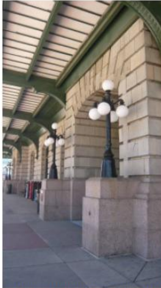
Figure 114: Detail view of typical terra cotta at the first floor level. Note that the terra cotta is laid in coursed ashlar with deep reveals. The surrounds at the first floor window and door openings have a lower reveal to create a flat field.
