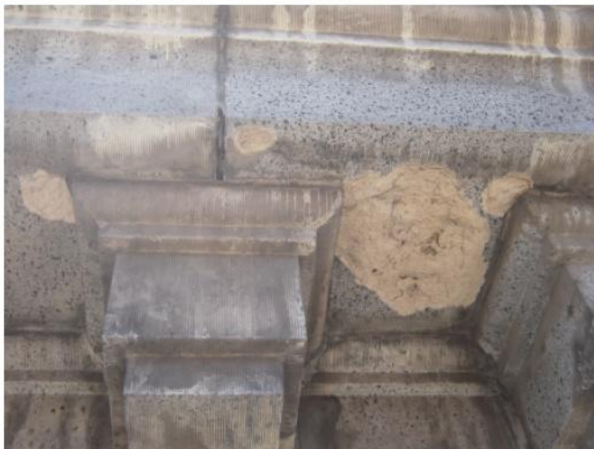
Figure 132: Detail view of open joints, terra cotta patches, and staining at the upper cornice of the central wing of the building.
