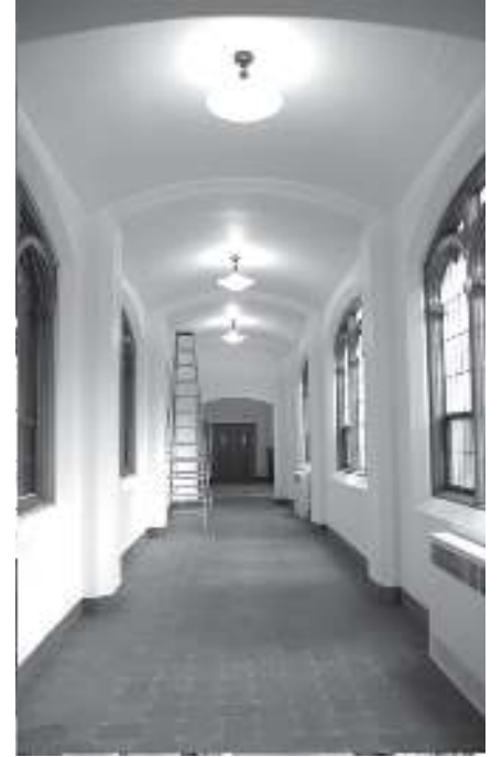
The flat plaster and windows in Miller Center hallway after restoration. Photos: Shannon Stage
