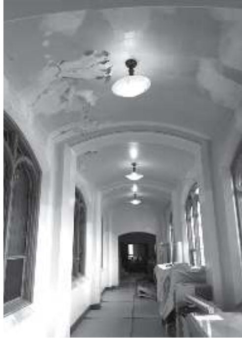
Deterioration of the plaster and windows in the hallway at Miller Center.
